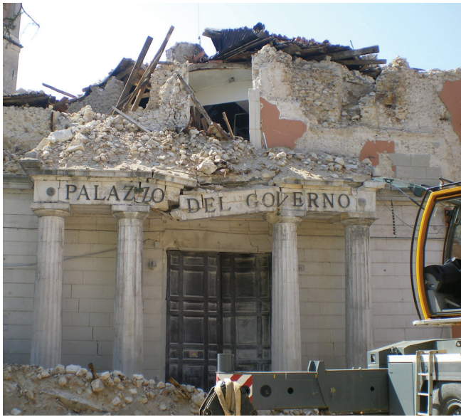
Aftermath of the 2009 L'Aquila earthquake. Image credit: TheWiz83/ CC-BY-SA-3.0
